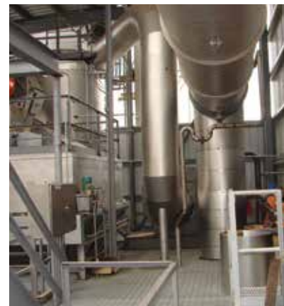
Product Cooler Mezzanine
