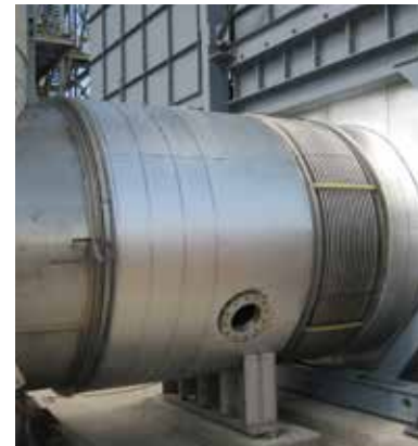
Steam Inlet to Hot Box
